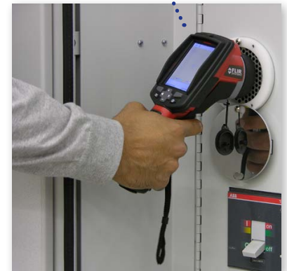
IR Portholes Allow The Operator To Keep The Deadfront Closed During The IR Scan Operation
