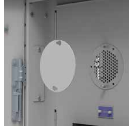
INSIGHT IR® Portholes allow operators to safely scan bolted connections without opening the dead front doors
