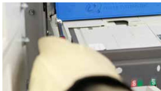
Screws Help Secure The Breaker
