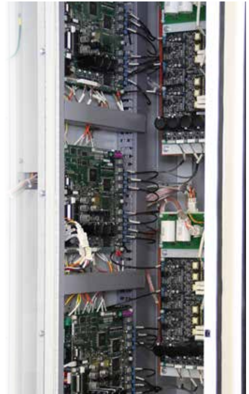
Three System Control Boards (SCBs) in a TMR Configuration
