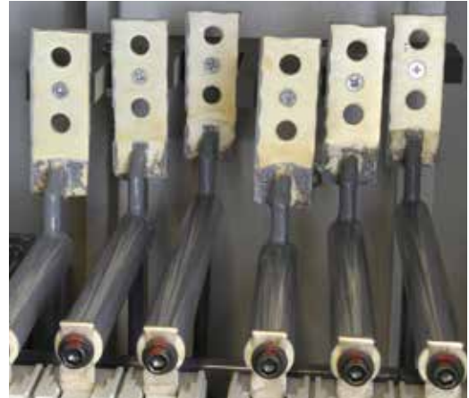
Silver-Plated, Epoxy Coated Customer Inputs for Source 1 and Source 2
