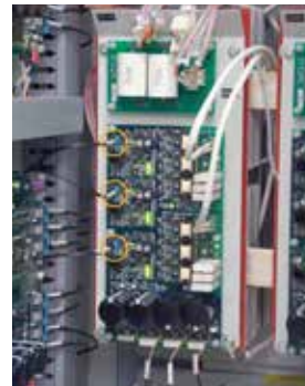
Fiber Optic Connections (highlighted) in a Gate Drive
