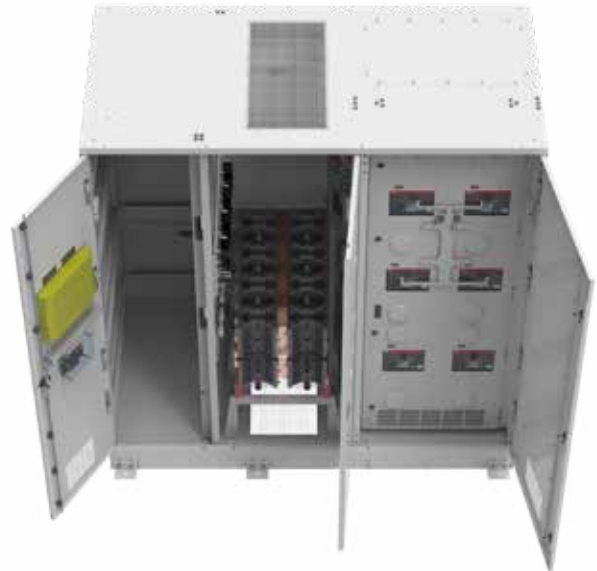
eSTS with the Outer Doors Open, showing physical separation between the power electronics and control sections
