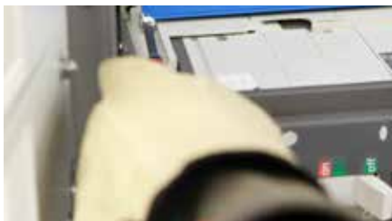
Screws Help Secure The Breaker
