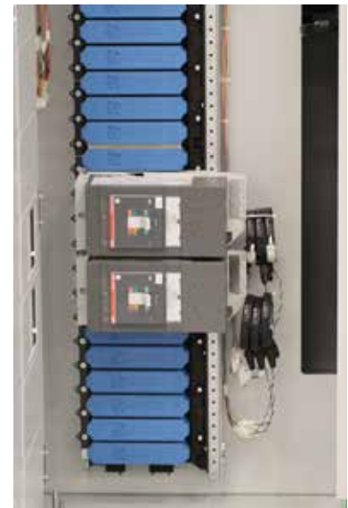
Two Subfeeds in the 1200 A SafePanel
