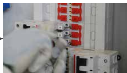
The Breaker Is Secured With An Isolated, Non Conducting Screw
