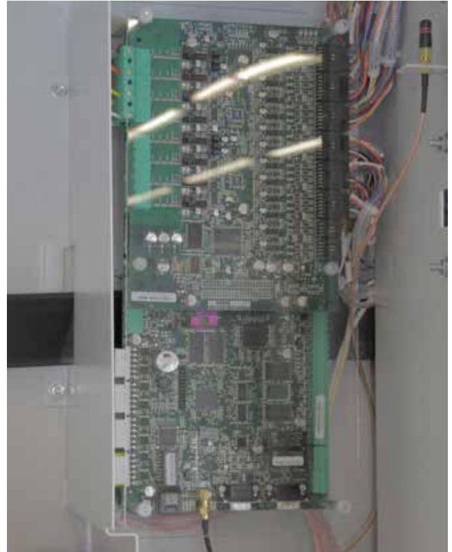
Serialized Panel Board Monitor (PBM) in an ePanel-2 Power Panel
