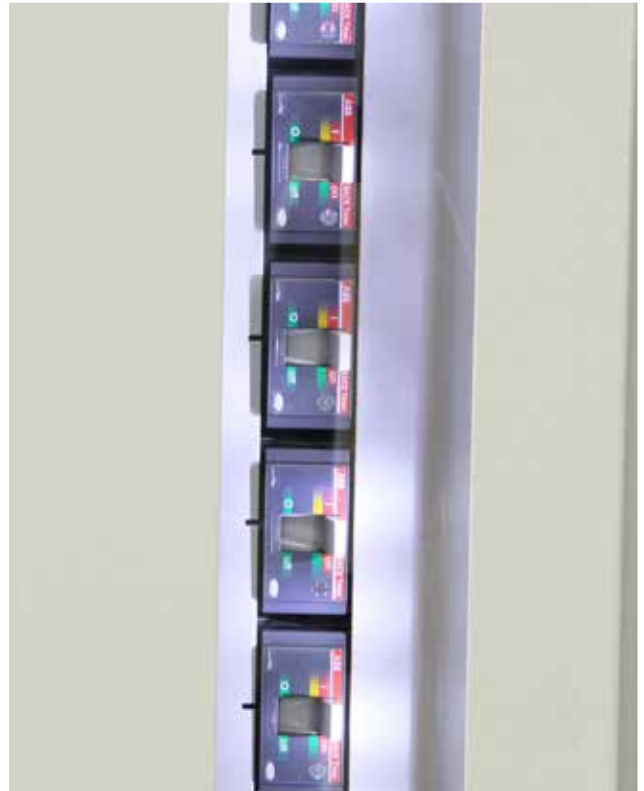
High-Density Power Panel Circuit Breakers
