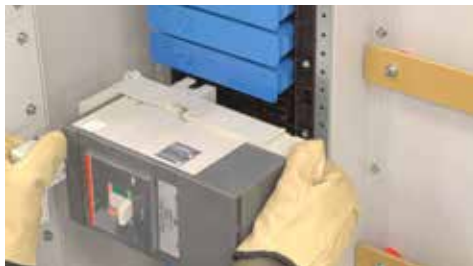
The Breaker Is Inserted Into The SafePanel
