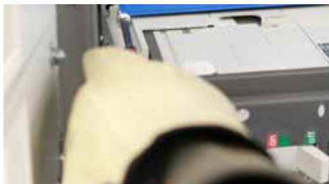
Screws Help Secure The Breaker
