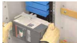
The Breaker Is Inserted Into The SafePanel
