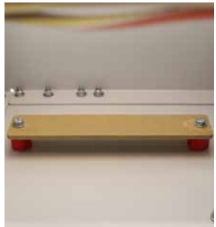
Guided Wireways help keep cables organized
