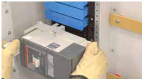
The Breaker Is Inserted Into The SafePanel
